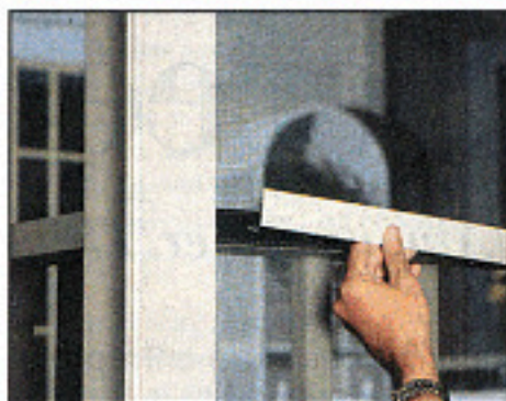
Screen-Tight utilizes an ingenious two-part system (top) that holds the screen in place. The screen is rolled into place with spline and a screen roller (center). A trim-piece cap, available in different colors, snaps onto the base strip. Screening a porch (opposite) becomes a breeze.
