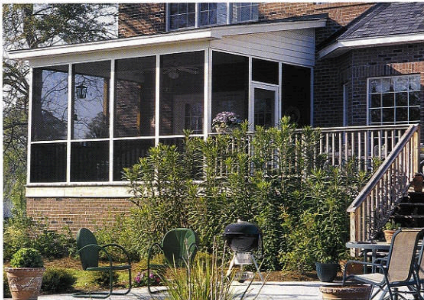
SCREEN STAR: THIS RENOVATED PORCH SPORTS all new screening installed with a low-maintenance vinyl track system.
