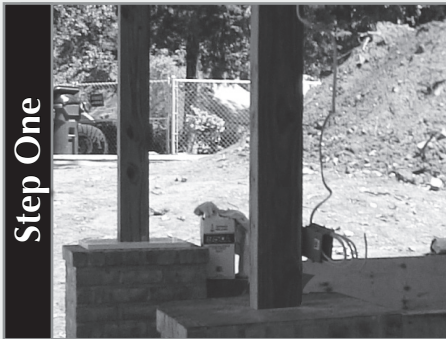
Step One Measure the height of the tapered column and cut to length if necessary.
